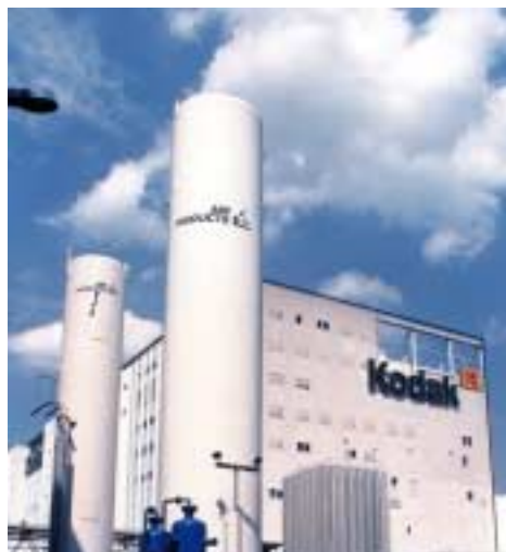
Figure 27. Typical On-site High-Purity Nitrogen (HPN) installation.
